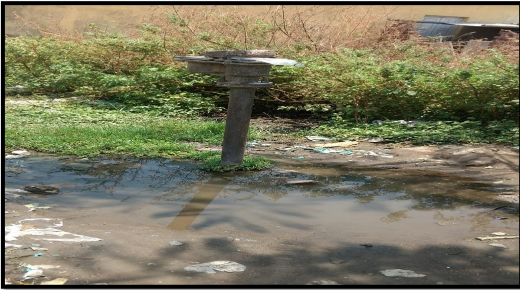
Plate: 2.3 The open water valves of the public water supply pipeline
