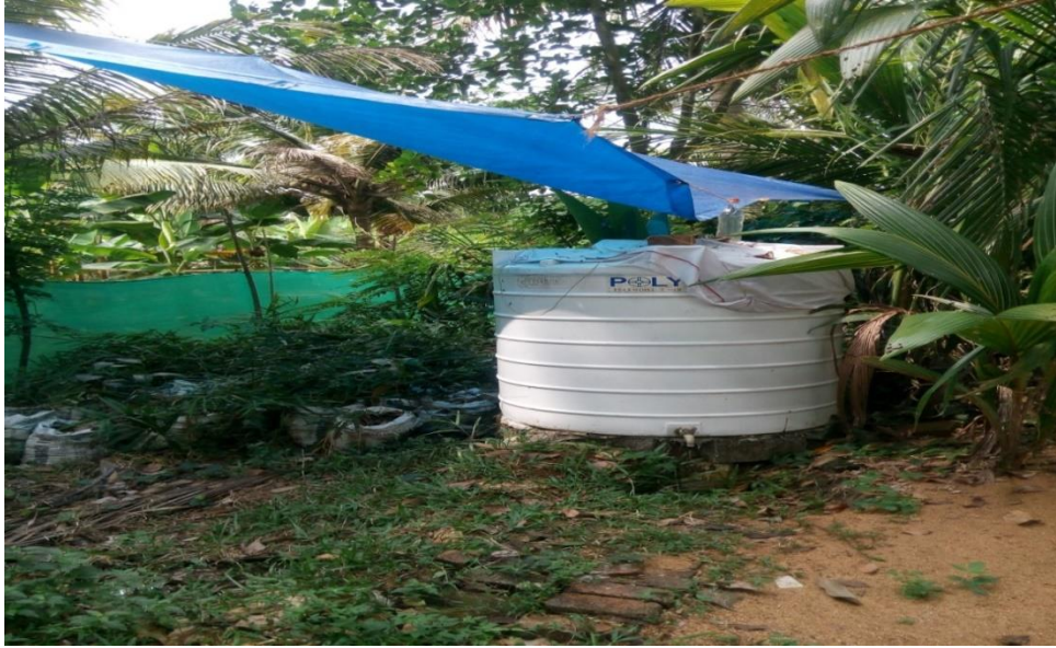
Photo 5.1: Rain water harvesting in the Puthukary village
