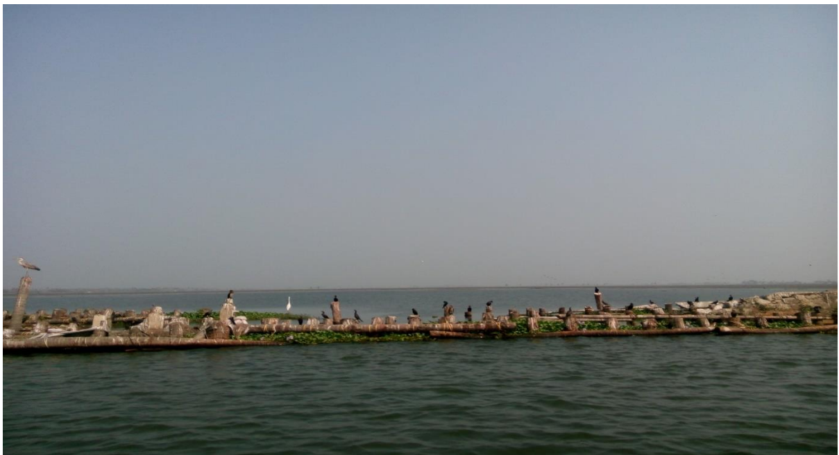
Photo 3.2: Damage to the bund in a kayal land
