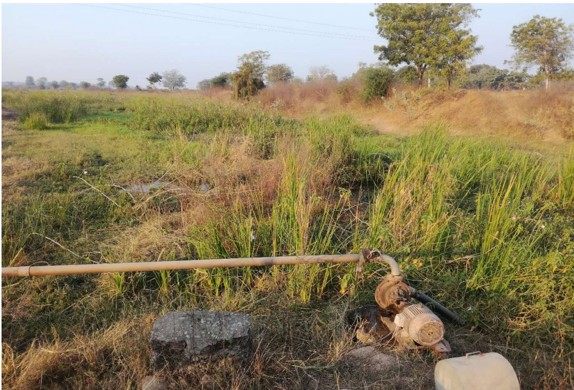
Figure 6: A view of Lift motor connected to leakage canal.
