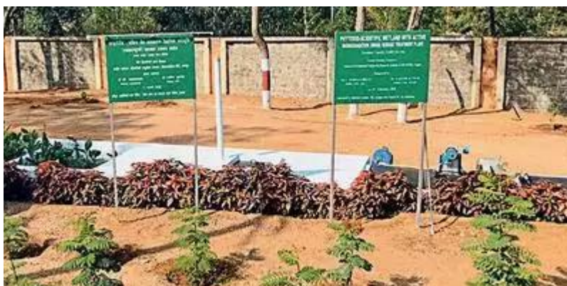
Fig. 6.1 Phytorid sewage treatment plant of 15 KLD established at ARCI by CSIR-NEERI
