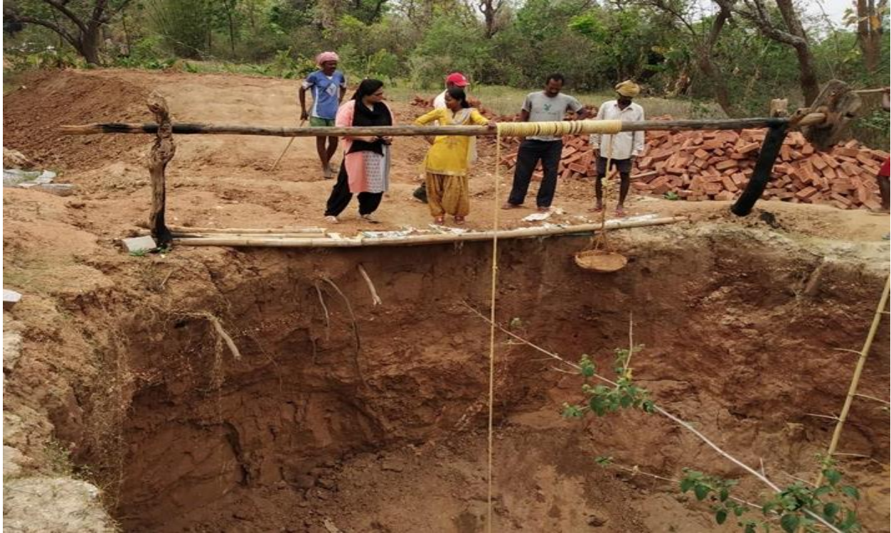
Picture 1: Workers showing an incomplete well, the construction of whose is on halt due to non-payment of material costs.
