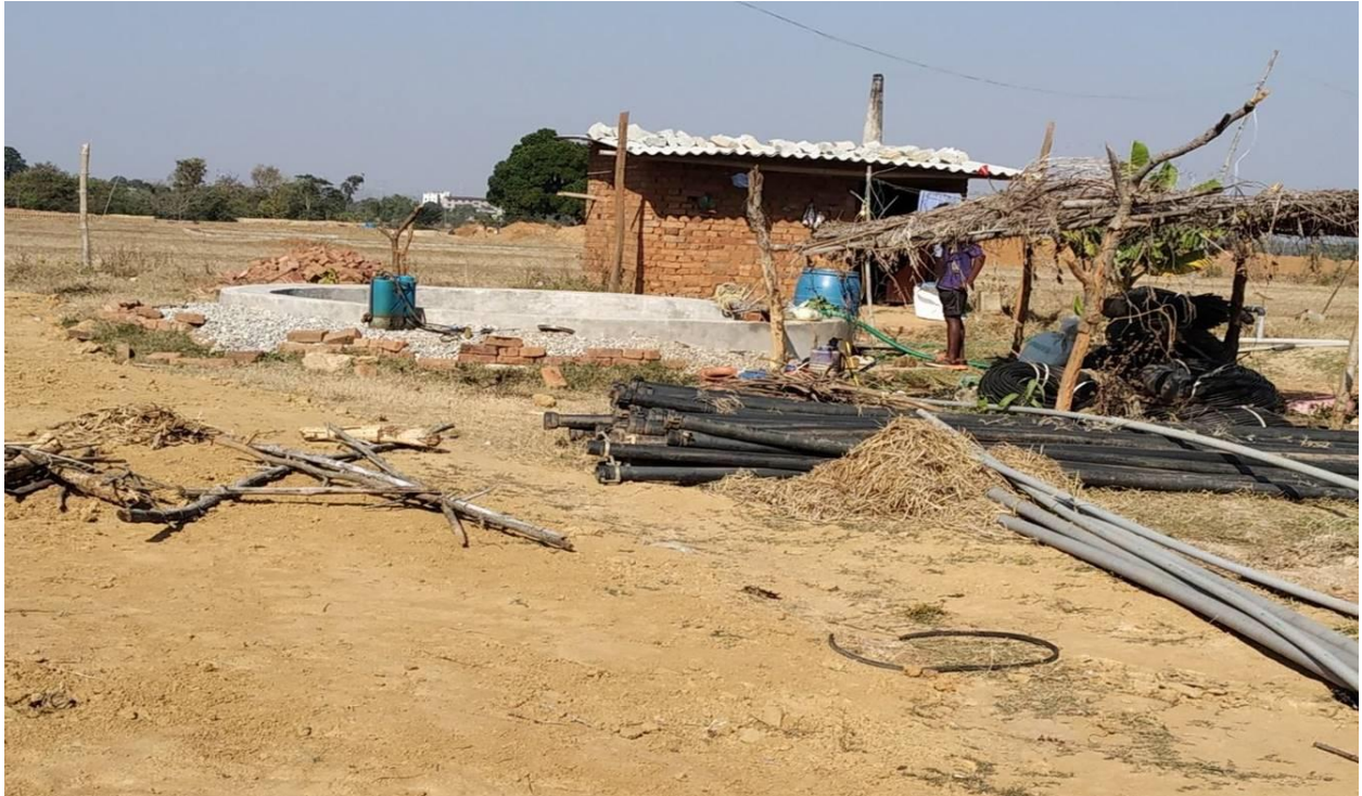
Picture 5: A deserted worksite under MGNREGS where no worker wants to work under meager wages.
