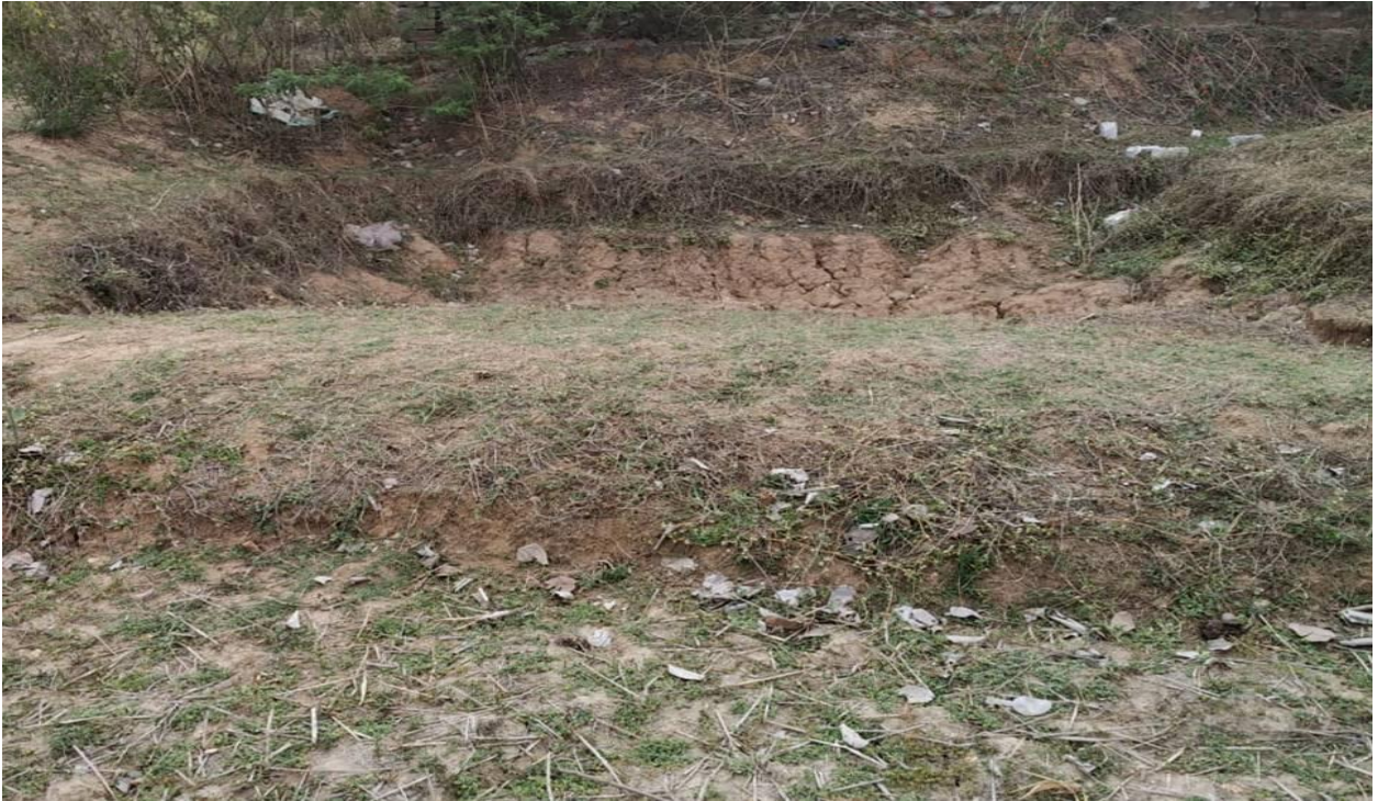
Picture 7: Dried up dobha (due to incomplete work).
