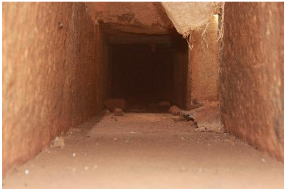
Plate 22 showing underground duct
