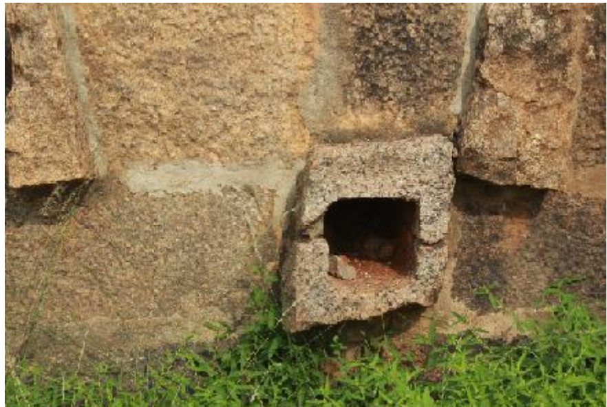
Plate 24, inlet of the tank
